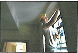
John Patriquin/Staff Photographer Sheet rocker Shawn Gosselin tapes a window inside a unit at The Olde Woolen Mill in North Berwick that is being converted into low income housing for the elderly.
